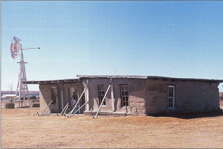
Before local opposition stopped destruction of the adobe house, the original pitched roof was removed. A flat roof was constructed during the first renovation effort.
