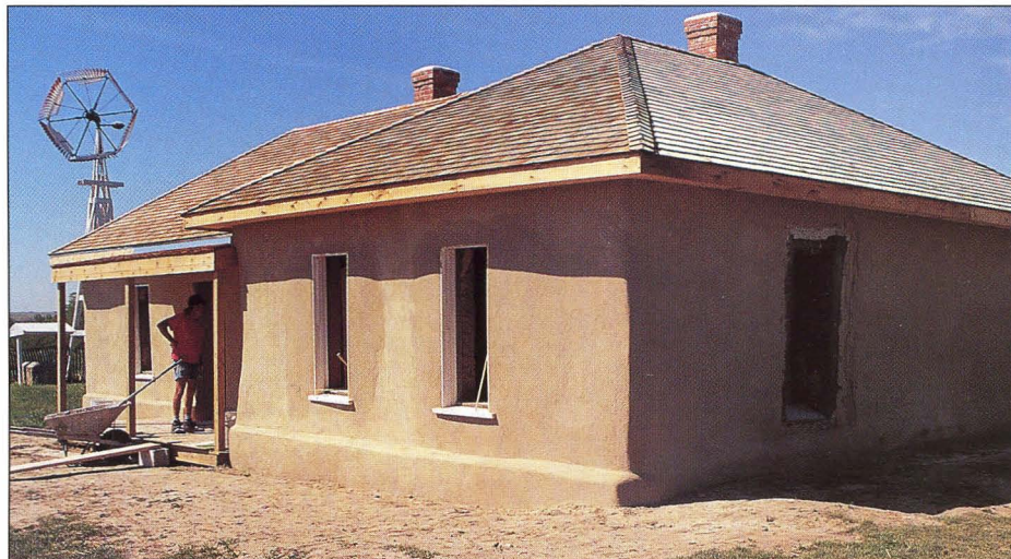
Using old photographs for reference, the recent renovation has returned the adobe house to its original appearance. A dedication is set for this spring.
