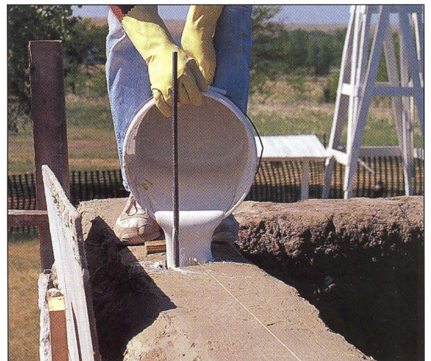
To stabilize original adobe walls, steel rods, which were connected to a new pitched roof, were epoxyed in.
